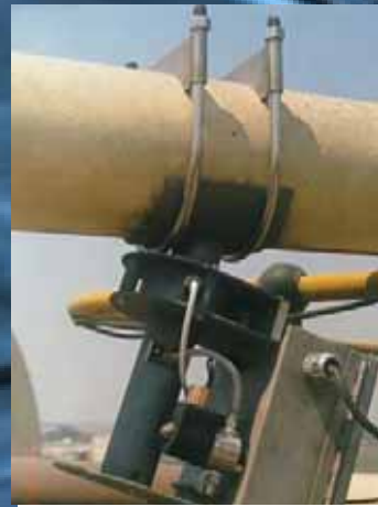
Pipeline Sampling Sensor
