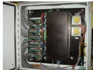
Data Concentrator adjacent to sensor array collects data and transmits to PC
